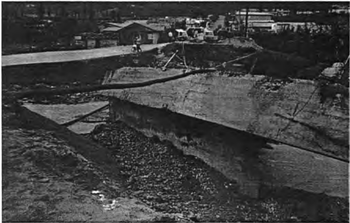
This bridge in Tireo Arriba, collapsed into the river as a result of storm damage. Debris removal began immediately in order to prevent further obstruction and a continued threat to loss of life and property. This is considered an exigency or urgent action.
