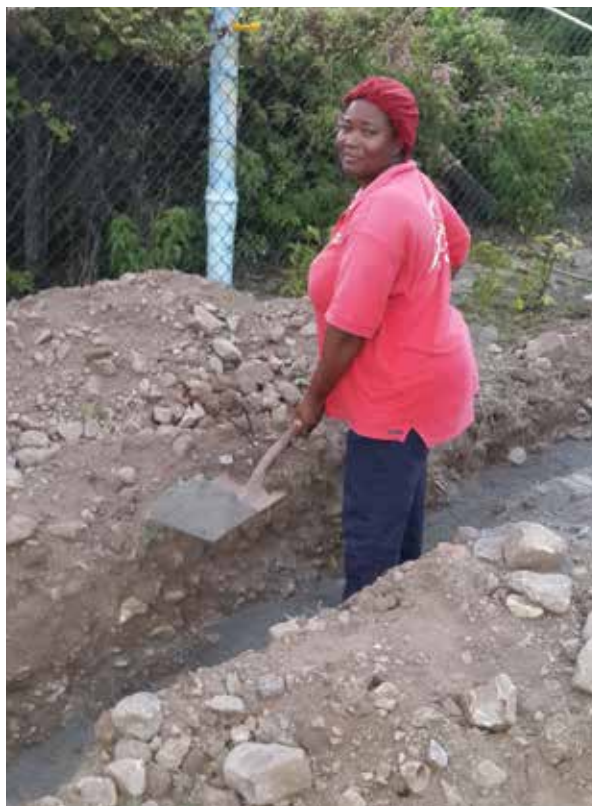
One of the Co-operative's female farmers Ms. Alana Leitch busy levelling off fill material along the trench.
