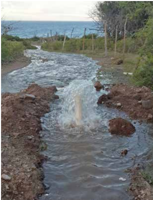
Flushing of pipe line to remove any debris before releasing water to farmers.
