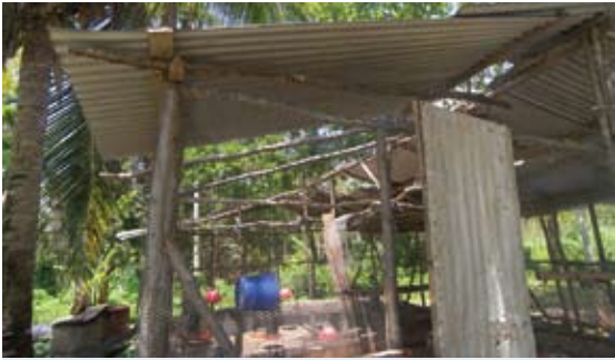
Damaged chicken coop in Mountain Pass, St. Catherine where 28 poultry operators benefited from the CIDA/IICA Hurricane Relief Programme.
