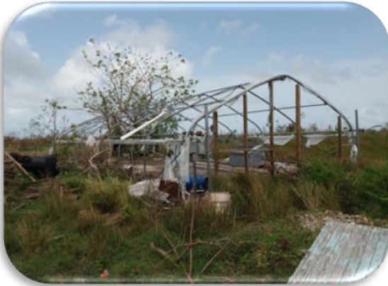
Greenhouse condition after the effect of Hurricane Irma
